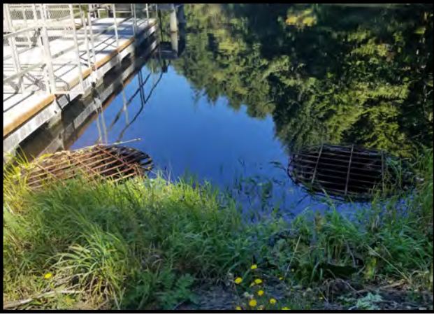
North Depoe Bay Reservoir outflow pipes as viewed from the dam.
